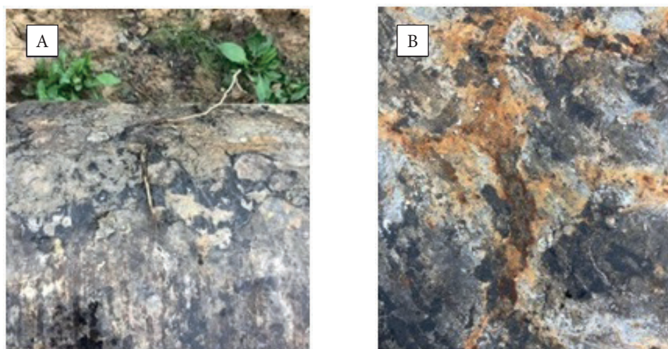
Fig. 1. Degradation of insulating coating (A) and metal damage (B) of main gas pipeline
